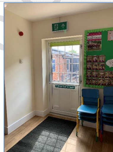
Figure 02 – The canteen doors that are not shutting correctly
