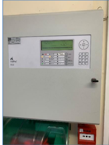
Figure 06 - The faults on the fire alarm that must be cleared
