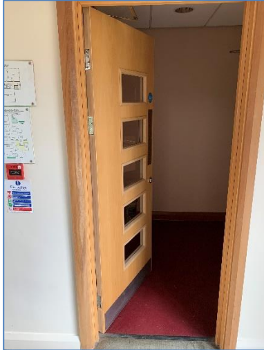
Figure 05 - The fire door from the balcony in Mundell building that is not closing correctly
